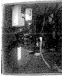
Control components in a clear and easily accessible main panel (p. 44). The top-hinged door provides shelter from snow/rain.
